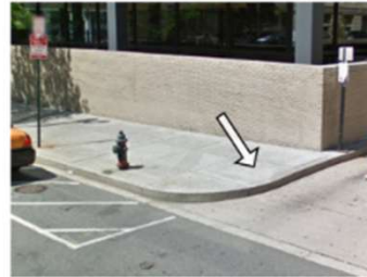
Missing Curb Ramps
